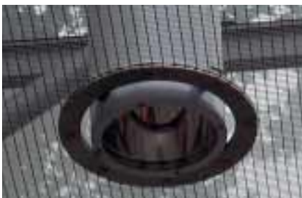
Detail showing integrated lighting
